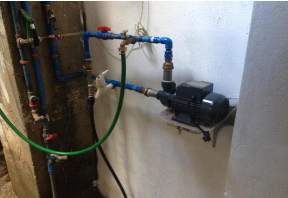
Booster water pump
