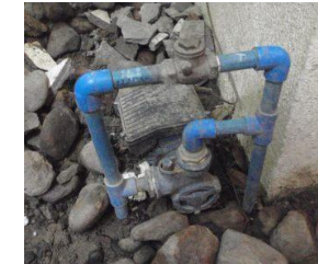
Booster pump and piping
