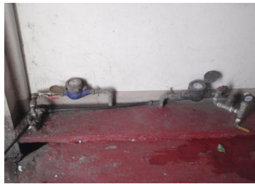
Two water meters in garage
