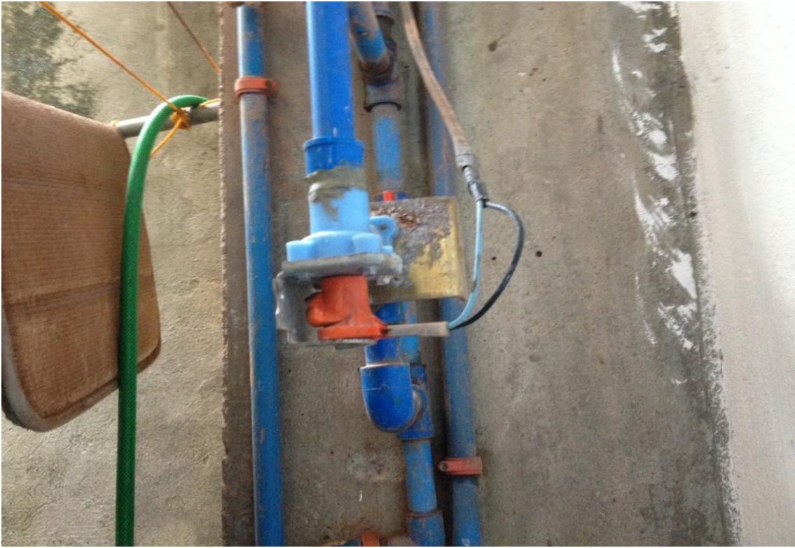
Solenoid valve for water tank fill line
