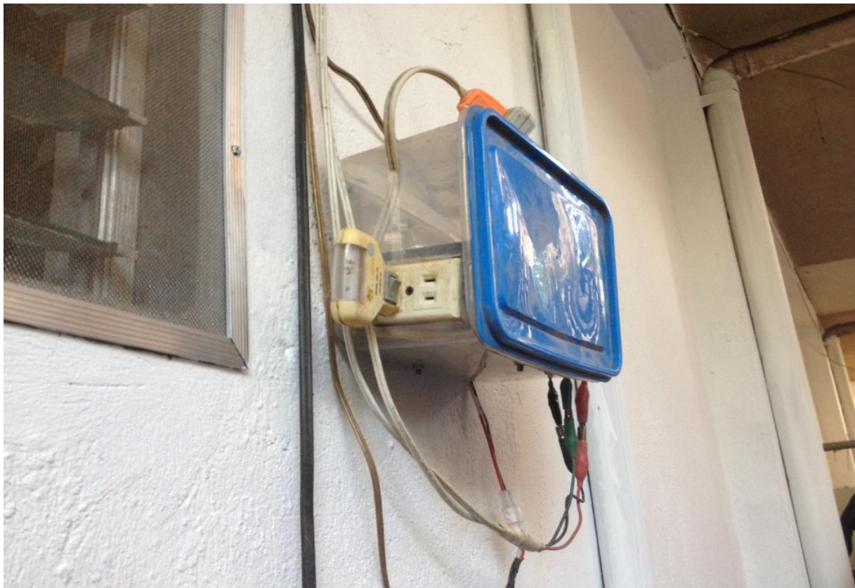
Plastic box protecting 12 vdc power supply and wiring
