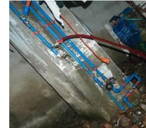
Pipes/valving on tank pylon
