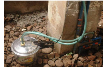
Pressure cooker as enclosure for solar fish-tank pump, 15 watt
