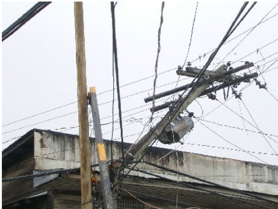
During the 4 days the Lakbayans were in Negros, portions of Metro Manila had no power due to the storm. The day after they left, Tanjay had no power for almost a day. At first I thought it was caused by a freak wind gust on that downed transformer above, and even text'd Mercy that they brought the bad weather, but I later found out it was a truck accident.
