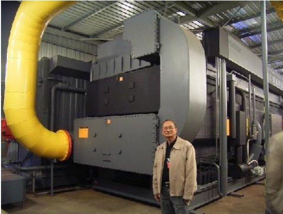
Me and the Broad – chiller.
